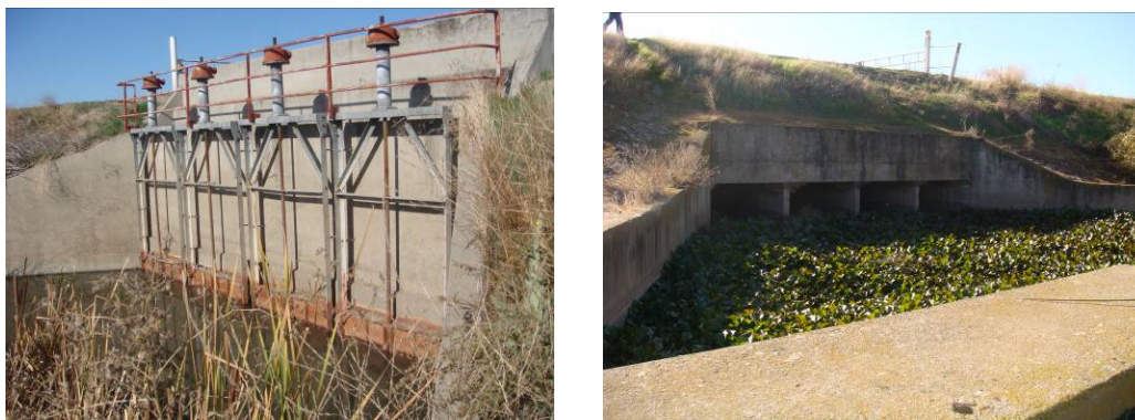
13 14 Figure 5-12. 15 Reach 4B Headgate
