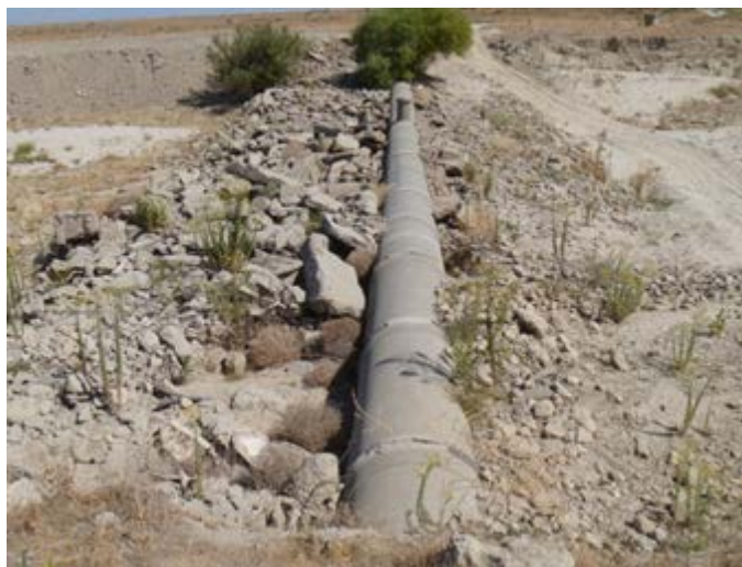
Pipeline in the Eastside Bypass looking east
